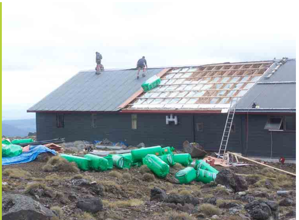
Installing the new roof on the Club Lodge Photo: Ken Mercer Lodge Re-Roofing Work Party 3-4 February 2007
